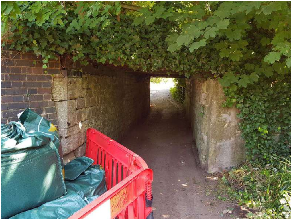
The Picture above shows the implementation of emergency gravel bags to hold up the deteriorating bridge wall.
